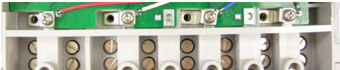
• Figure 7-12 Meter with the CT to VT links disconnected by removing screws.
