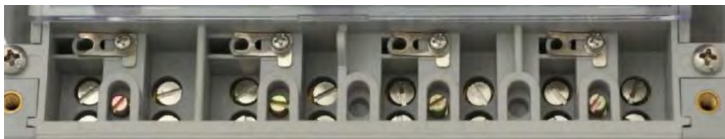
Figure 3-10 Meter with the CT to VT links disconnected by removing screws.
