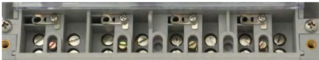
Figure 7-10 Meter with the CT to VT links disconnected by removing screws.
