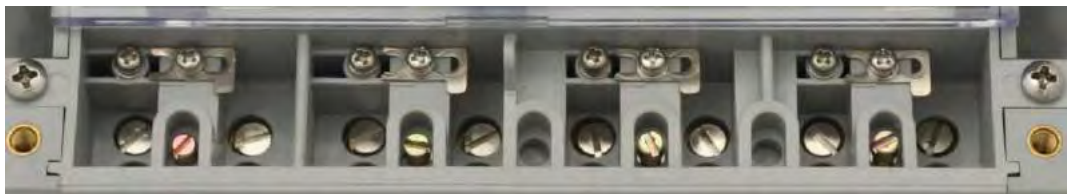
Figure 7-9 Meter with the CT to VT links disconnected by sliding shims.
